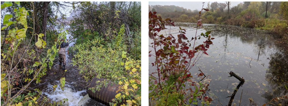
Outlet culvert of CSA 1a (left) and area around CSA 1b (right) with tiered vegetation.
