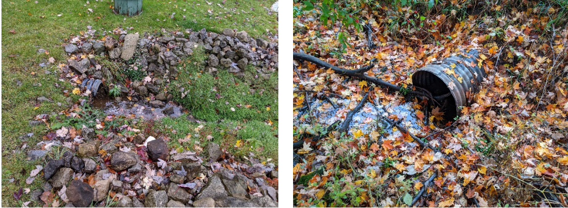
Outlet culvert of CSA 4a (left) and CSA 4b (right)
