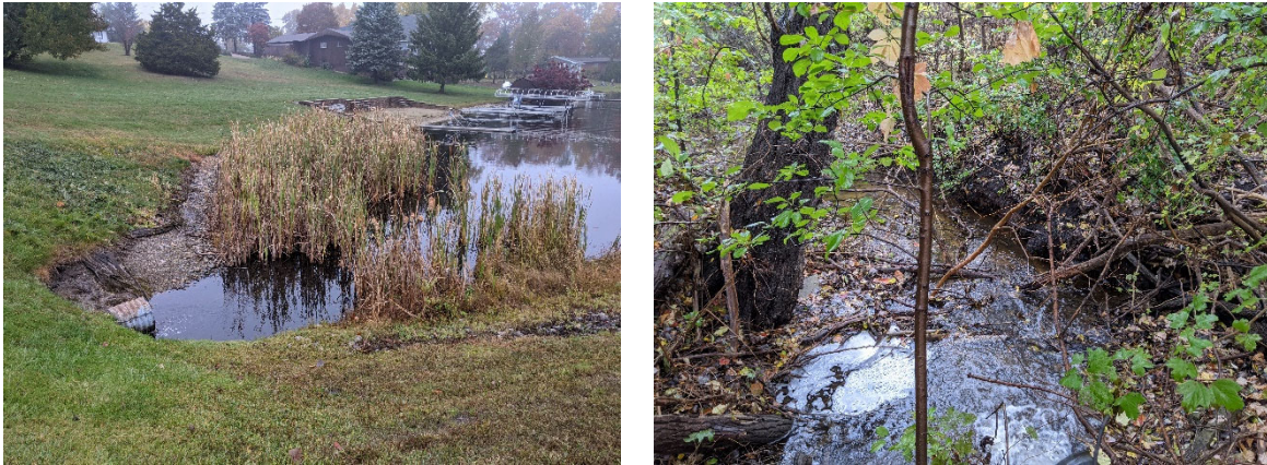
Outlet culvert of CSA 2a (left) and eroding stream bank of CSA 2b (right).
